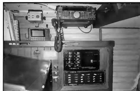
The GPS, radar detector and ham radio above with the breaker panels below
