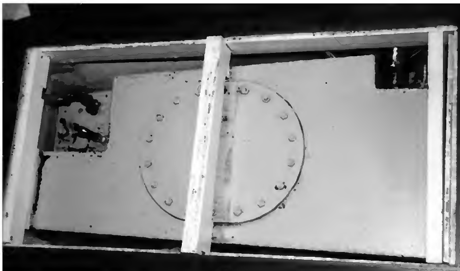
This tank doesn't look too bad, does it?
